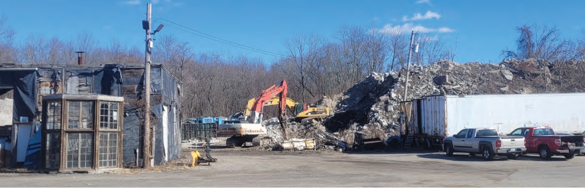
TOO BIG TO STAY: AA Wrecking & Asbestos has been operating at 1307 Hartford Ave. since 1986. The business has outgrown the site, nestled in the heart of Johnston's business district, next to the Johnston Senior Center and across the street from Market Basket. The business may be moving and a new business may be moving in. (Sun Rise photos by Rory Schuler)
